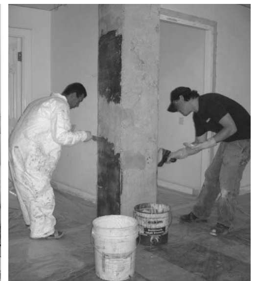
Tyler Maas, of the California-based Fyfe Co., instructs the Armenian crew in seismically reinforcing the building.
