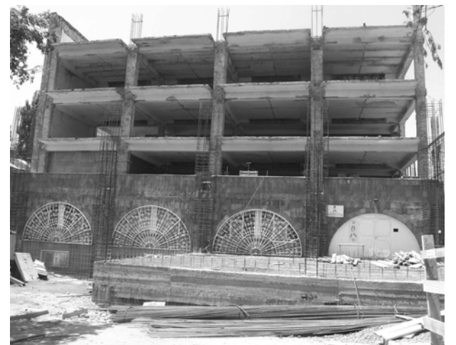
The Wellness Center as it looks today, in the process of a major renovation project which includes seismic reinforcement and expansion.
